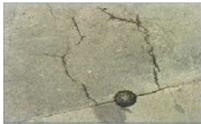
Fig. Cracking in topping concrete.
