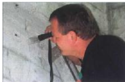
Fig. Measurement of crack in concrete.
