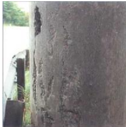
Fig. Pier with corroded reinforcement.
