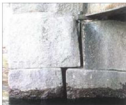
Fig. Movement in pier.
