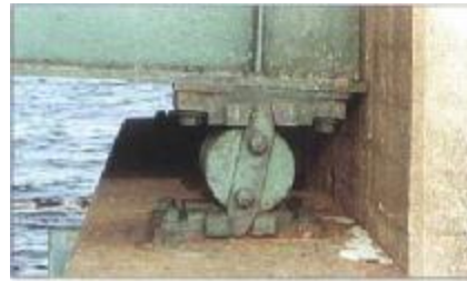
Fig. Contact with the ballast wall may cause deformation in a steel girder.
