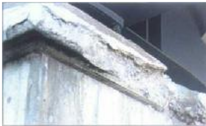
Fig. Weathered concrete on bearing seat and breast wall.
