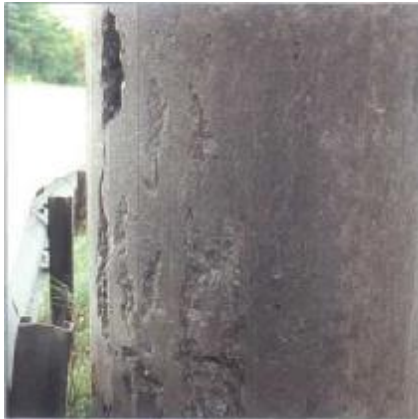
Fig. Pier with corroded reinforcement.
