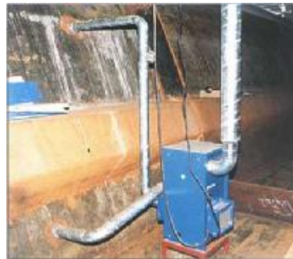
Fig. Dehumidification apparatus inside a steel box girder
