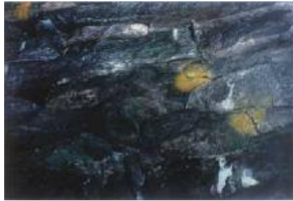
Fig. Cracked stones on the intrados.
