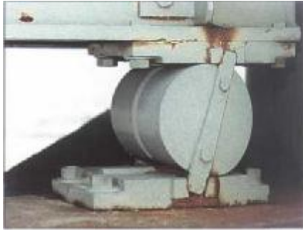
Fig. Misaligned bearing.
