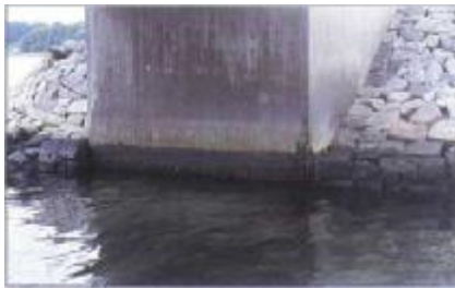
Fig. Weathering of concrete on the abutment.
