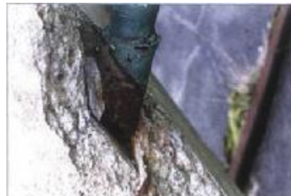
Fig. Corrosion of suspender.
