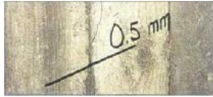
Fig. Tension crack on abutment breast wall.
