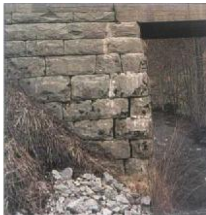
Fig. Movement in abutment.
