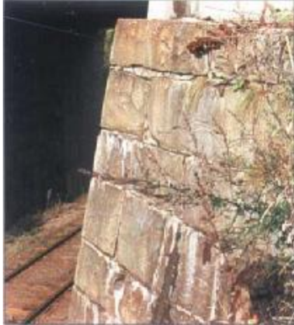
Fig. Weathered mortar.
