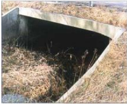
Fig. Blocked watercourse.
