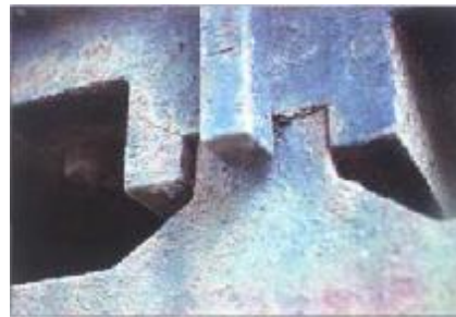
Fig. Crack on bearing.
