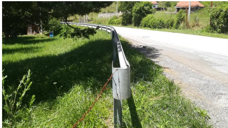
Picture 32. Part of the subject of the road near the elementary school "Dositej Obradovic" without sidewalks
