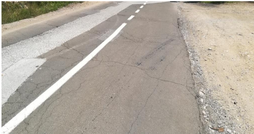
Picture 19. The example of damage to the subject section
