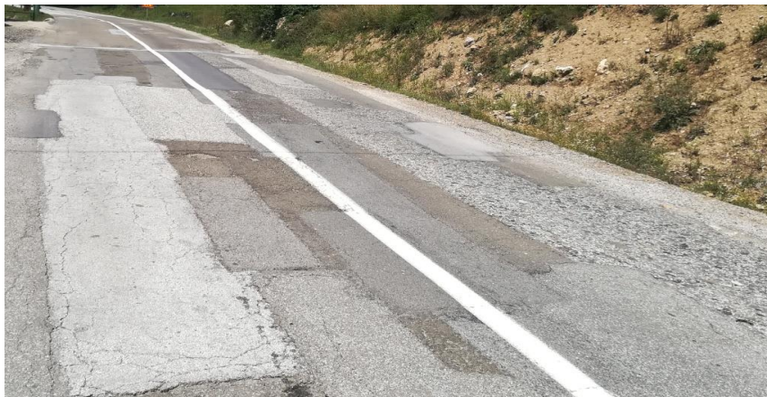
Picture 17. The example of damage to the subject section
