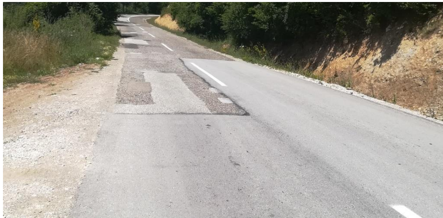
Picture 21. The example of damage to the subject section
