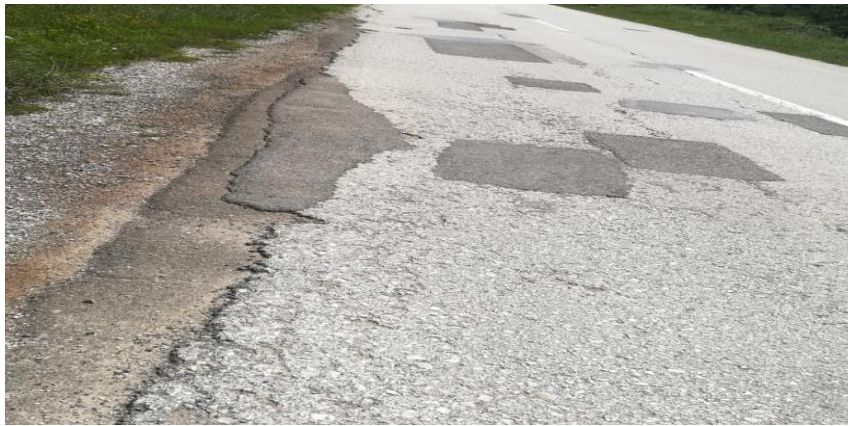
Picture 18. The example of damage to the subject section
