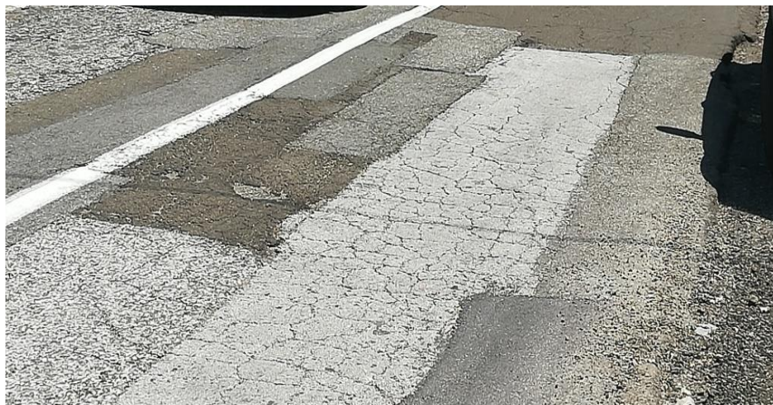
Picture 20. The example of damage to the subject section
