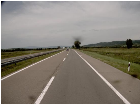
Picture 36. Damage of pavement
