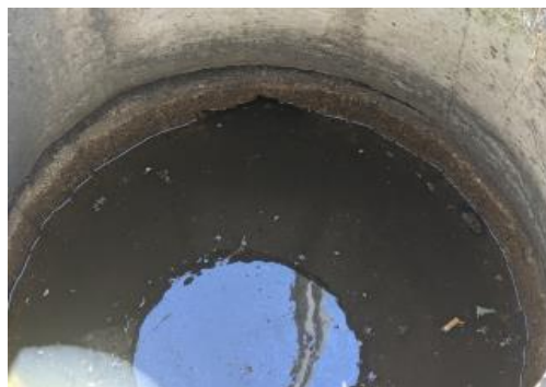
Picture 18 - Water retention in the manhole
