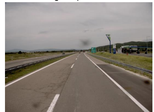
Picture 39. Damage of pavement
