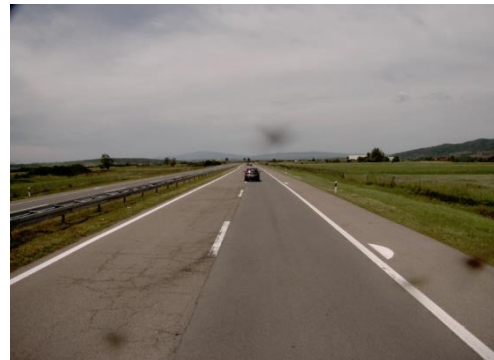
Picture 37. Damage of pavement
