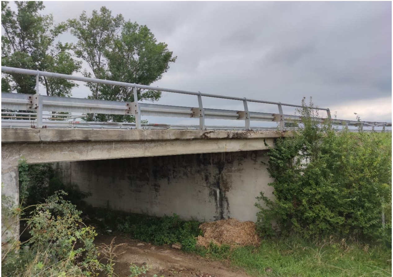
Picture 34- Bottom slopes overgrown by vegetation, unmaintained zone under the bridge, cornices damages
