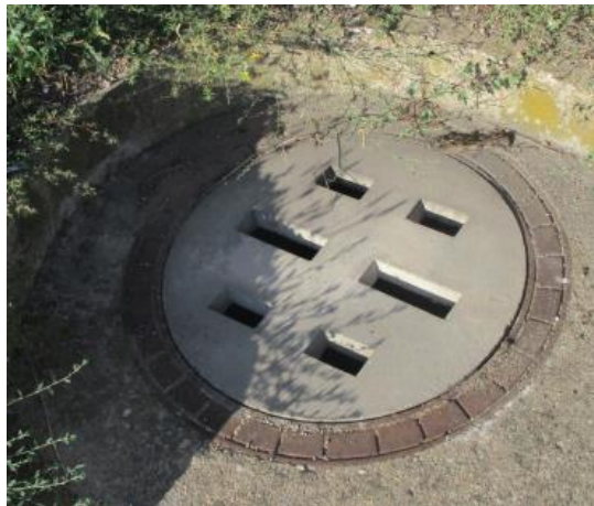
Picture 17 - Standard manhole with cover for water passage
