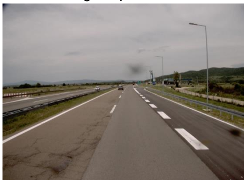
Picture 38. Damage of pavement
