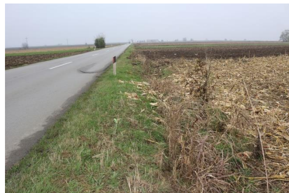
Figure 2-36 km ~25+500 irregular-shaped ditch, covered in vegetation, further it is turned into arable land
