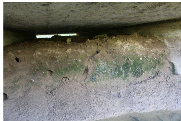
Figure 2-39km 30+498 culvert filled with material
