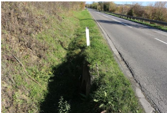
Figure 2-42 km ~27+100 the ditch of the irregular shape
