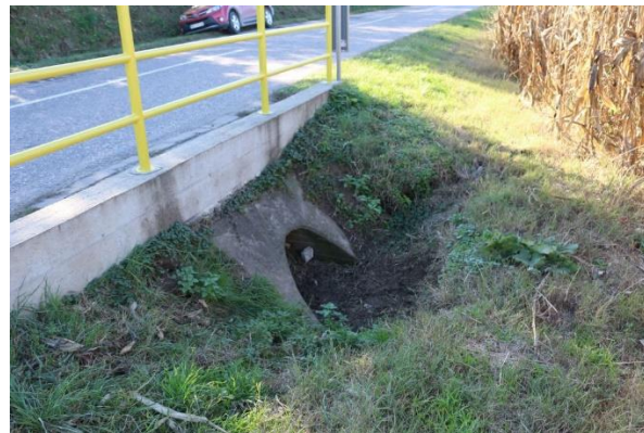
Figure 2-43 km ~30+650 no ditch prevents the culvert from functioning properly
