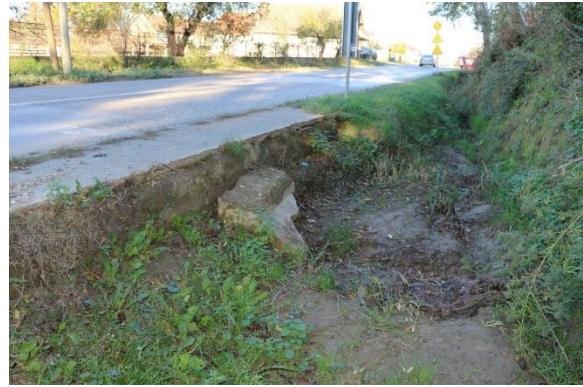
Figure 2-41 km 33+354 culvert filled with material, broken culvert head
