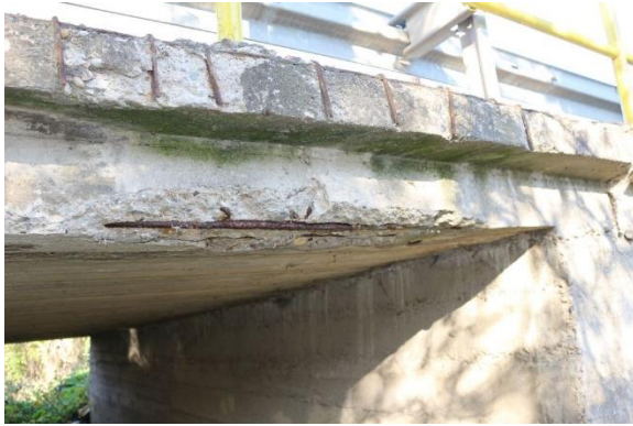
Figure 2-40 km 31+337 the protective plaster layer has fallen off
