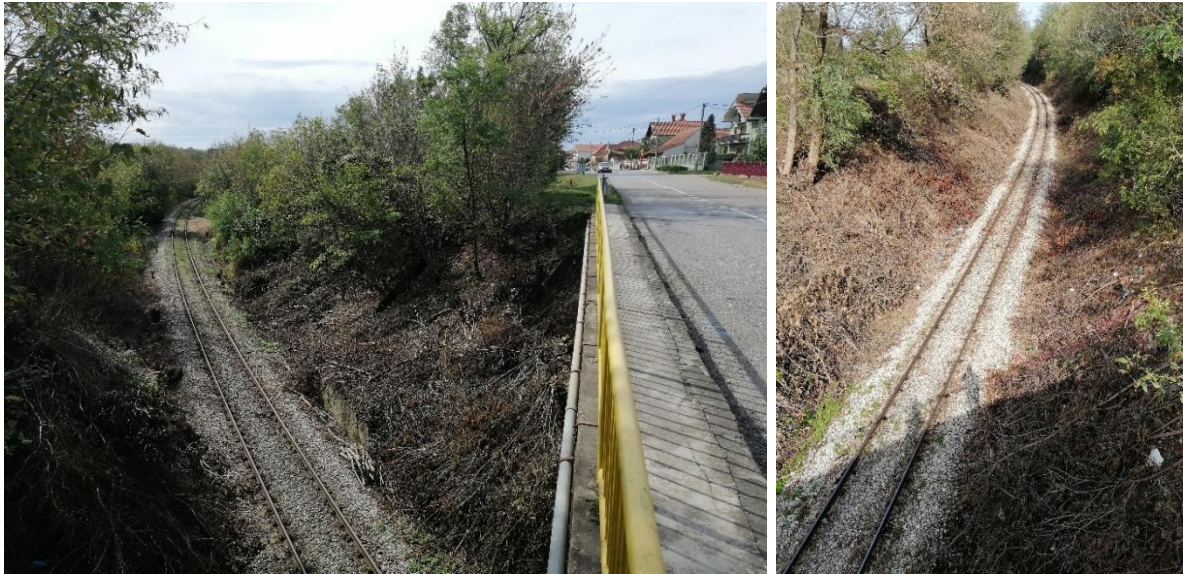
Figure 2-28 Unleveled crossing of the railway and the subject road section, Sirakovo at km 21+890
