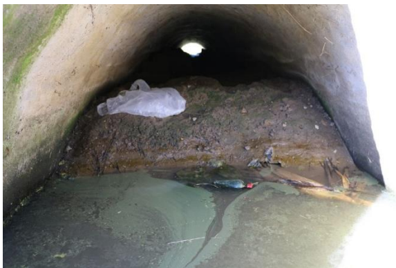
Figure 2-38 km 28+873 – culvert filled with material
