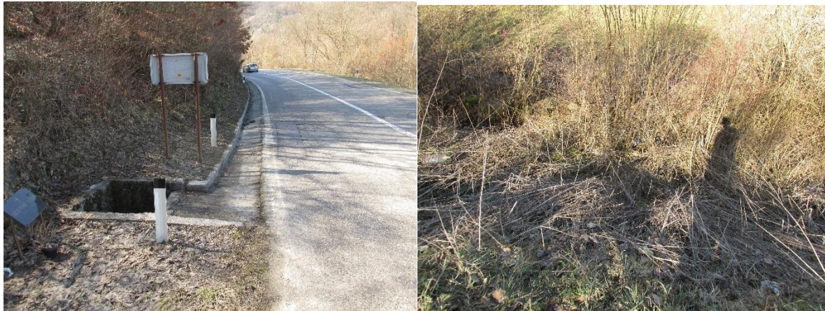
Figure 30. The inlet structure of pipe culvert that collects runoff from gutter, the outlet structure of culvert overgrown with vegetation
