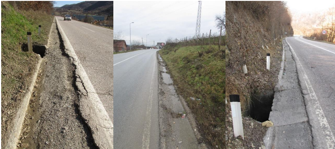
Figure 12. The gutter on the observed road section
