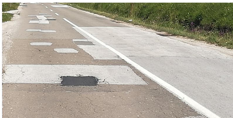
Picture 15. The example of damages on the section
