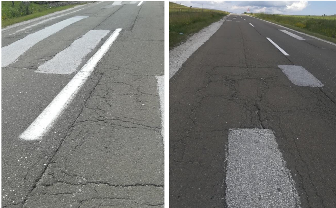
Pictures 13. and 14. The examples of damages on the subject section
