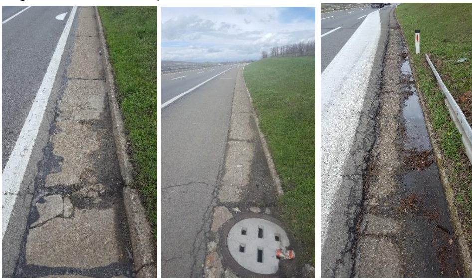
Figure 10. Gutters on the subject section
