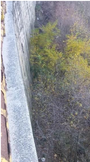
Figure 13: Example of the outflow of the road culvert in the retaining wall to the remote recipient
