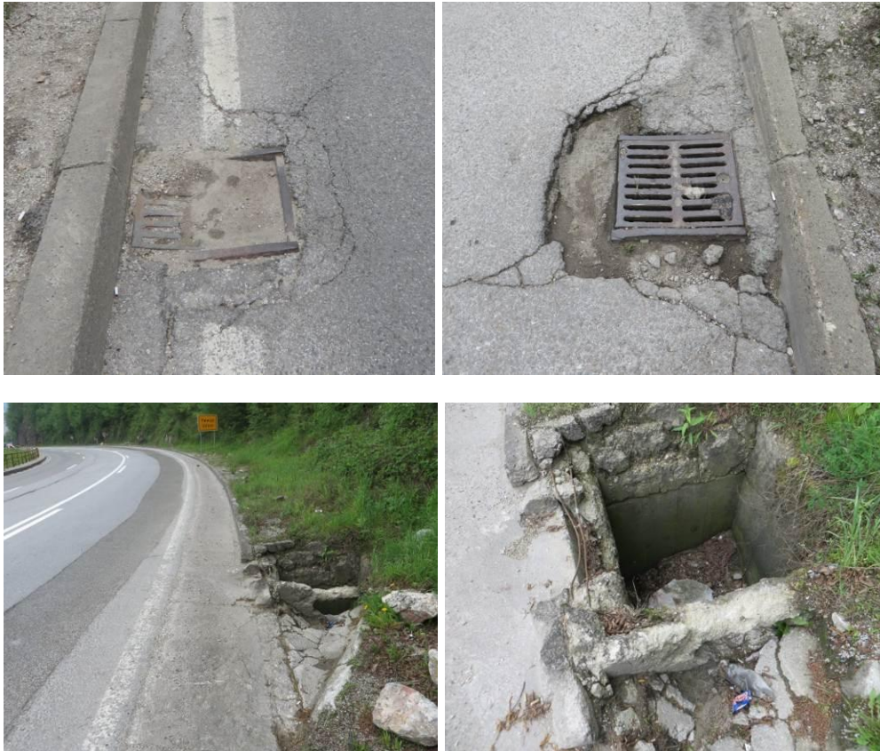
Figure 11. Damage to the drainage elements
