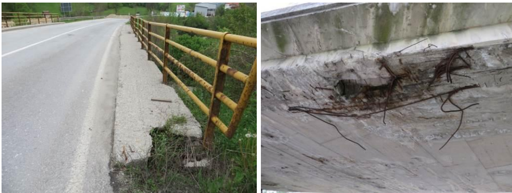
Figure 8. Damage of structures
