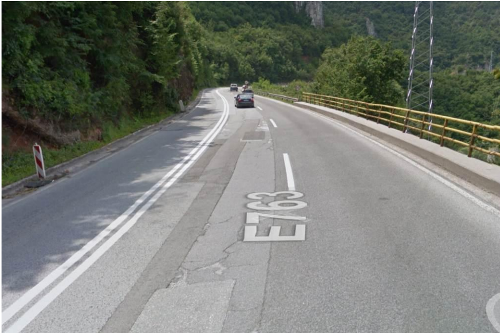
Figure 7. Example of damage of the road section
