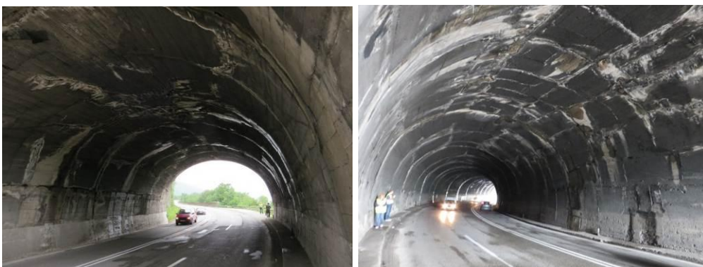
Figure 9. Damage to the lining of the tunnel
