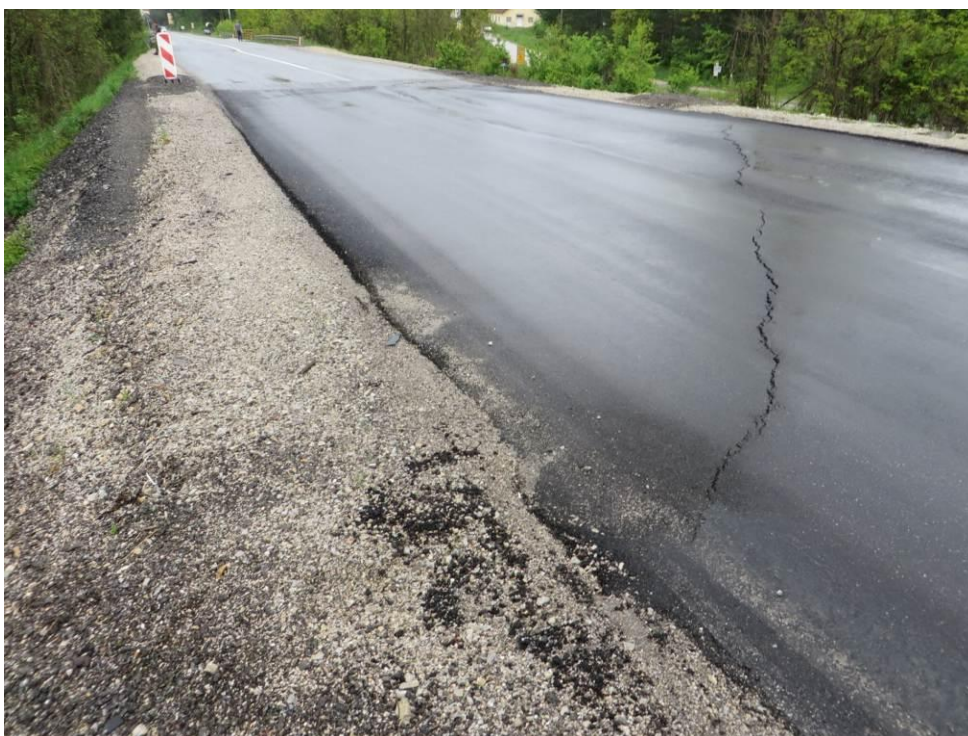
Figure 10. The deformation of the road
