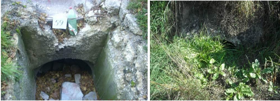
Figure 12: Example of reducing bandwidth of the culvert and need for rehabilitation
